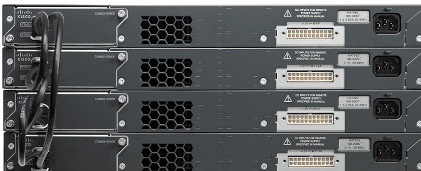
Figure 2. Cisco FlexStack-Plus Switch Stack
